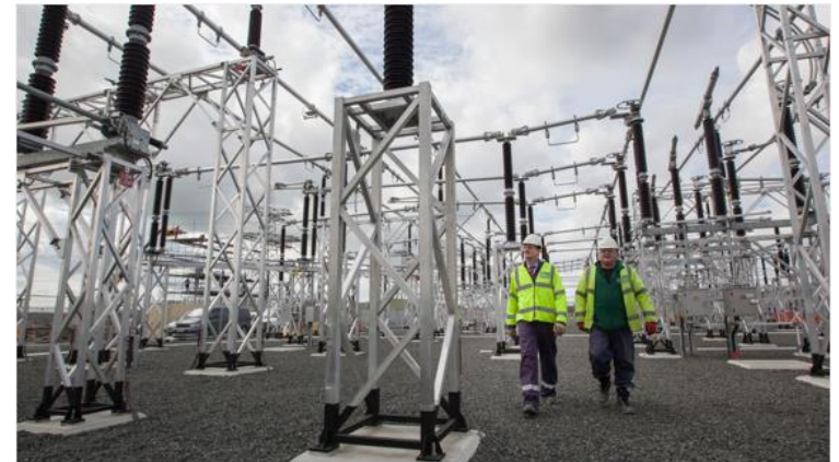
Beaulieu Denny Substation
